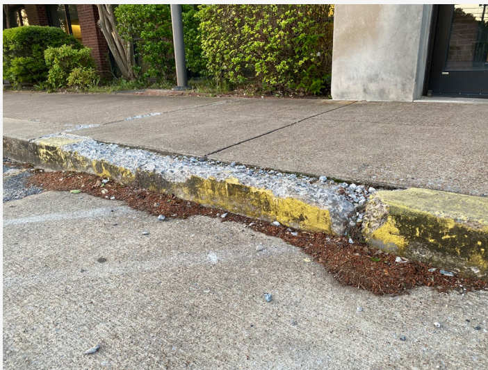
Figure 1. Crumbling Sidewalk Concrete
