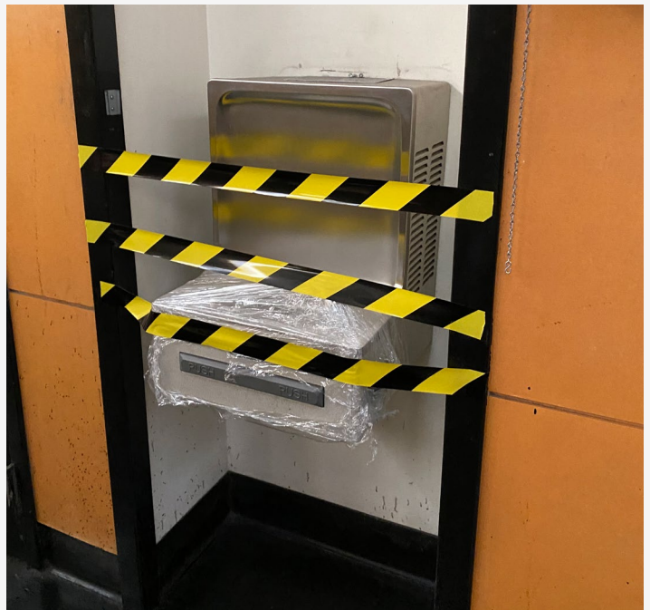
Figure 5. Non-Working Water Fountain
