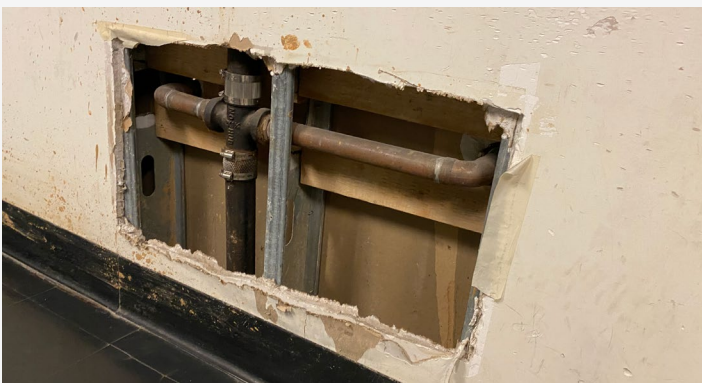
Figure 4. Men’s Bathroom Wall Damage
