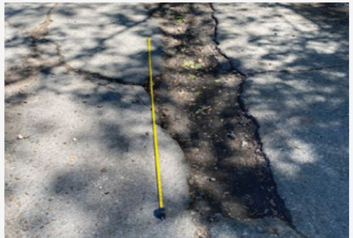
Figure 4. Large Potholes in the Rear Parking Lot
