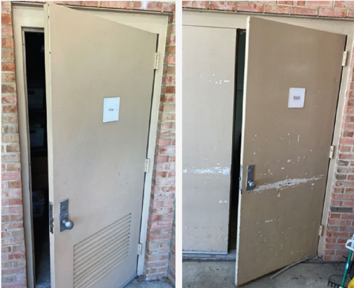
Figure 5. Doors to the Electrical/Furnace Room Could Not Be Locked
