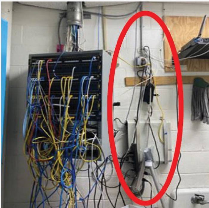
Figure 2. Multiple Cords in Server Room Plugged into Power Strips
