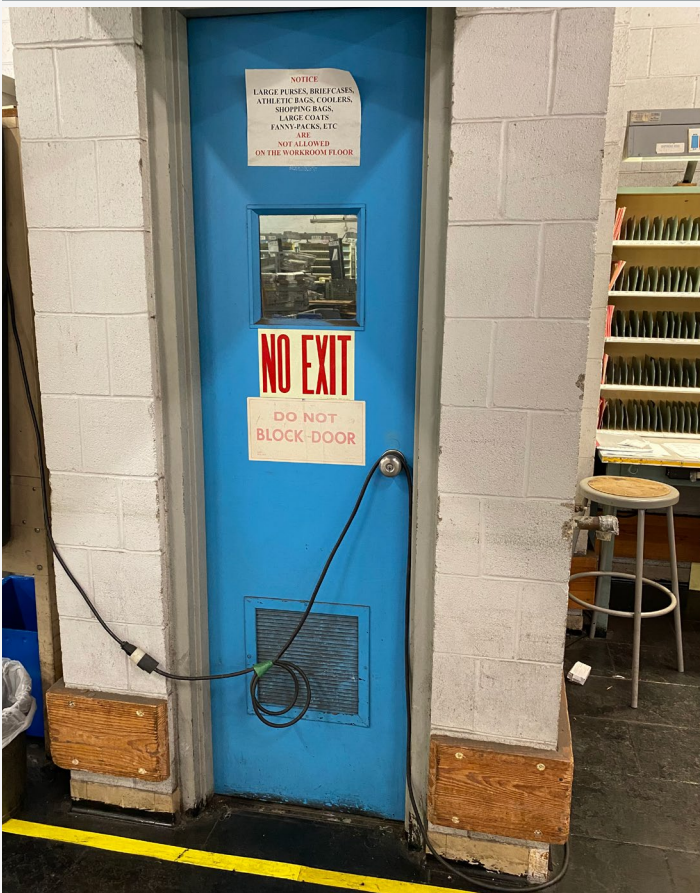
Figure 3. Blocked Inspection Door
