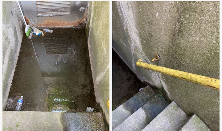
Figure 5. Standing Water and Damaged Handrail Outside Basement Door
