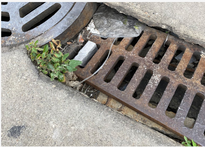
Figure 4. Misaligned Ground Plate in Parking Lot
