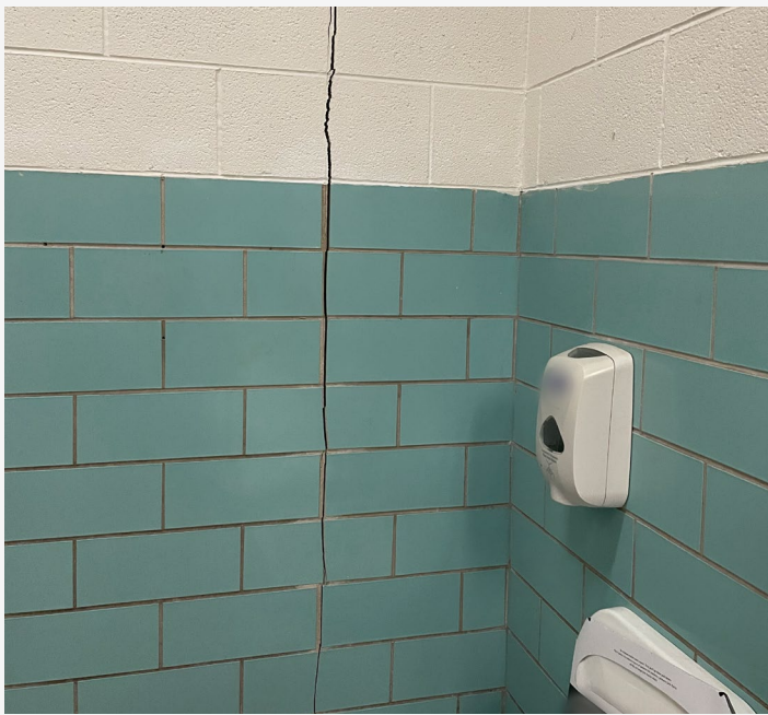
Figure 6. Crack on Wall in Men’s Restroom
