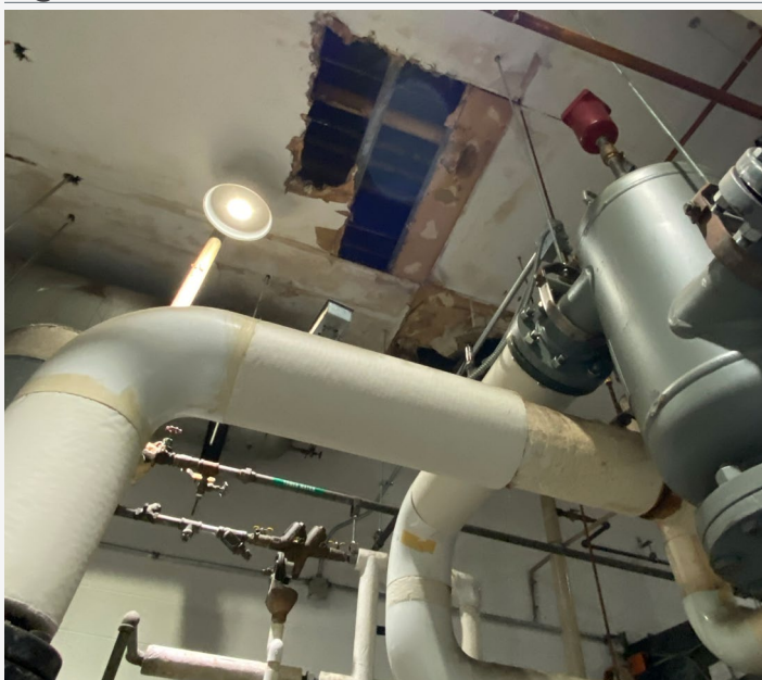
Figure 7. Roof Leak in Boiler Room
