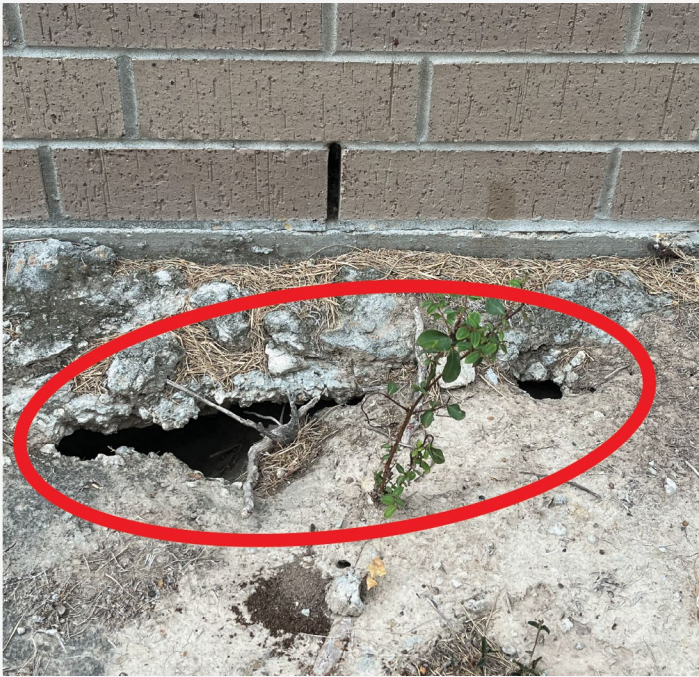
Figure 6. Hole in Front of Building
