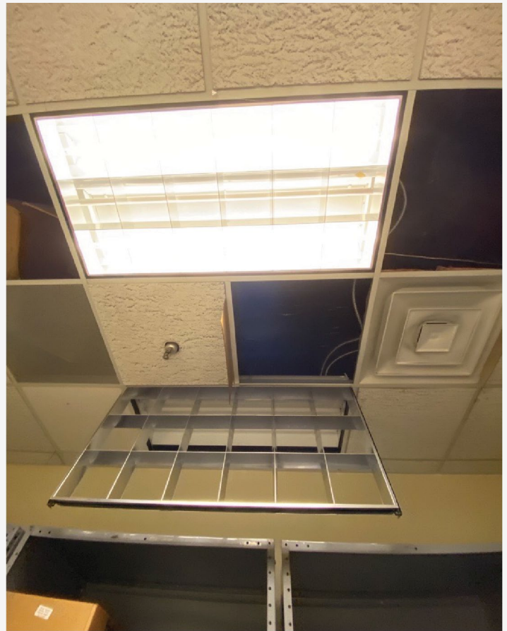
Figure 5. Missing Ceiling Tile in Storage Room
