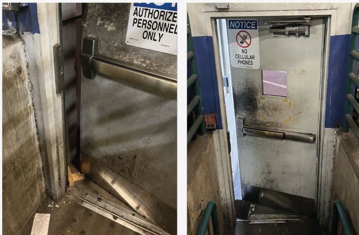
Figure 6. Propped Open Exit Doors
