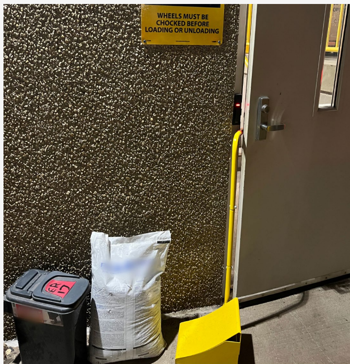
Figure 4. Wheel Chock Incorrectly Used as Door Prop
